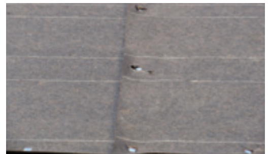
Standard felt tears and curls away from fasteners after exposed to moisture.
